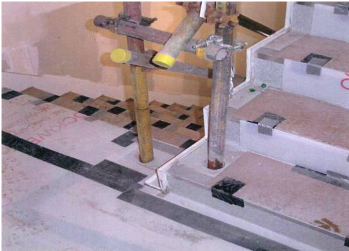
This photo shows cast sockets along the open side of a stairway, The sockets make it convenient to install temporary or permanent guardrails.
